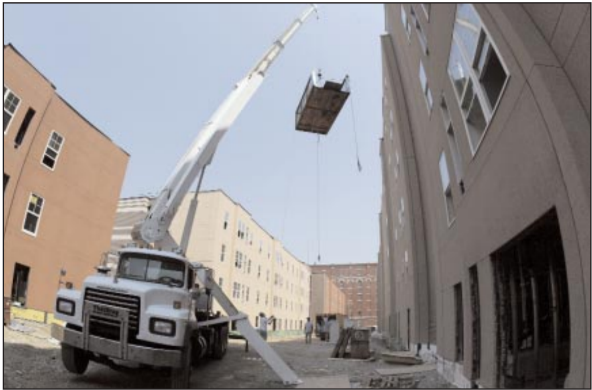
Construction crews add walls and windows to the University Village, a new residence hall at 10th Street between Cecil B. Moore and Montgomery avenues. The three-building facility, financed entirely through private equity, will open in time for the fall 2004 semester.
