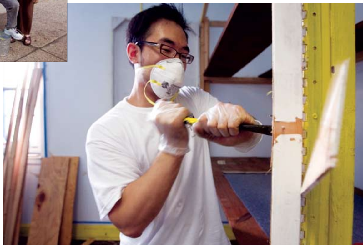
Demolition man: Temple Law student David Chung dismantles a cabinet at St. Boniface, an aging former church complex in nearby Kensington that's being redeveloped by a local non-profit, the Norris Square Community Association (NSCA). At the event are (inset above) are Professor Edward D. Ohlbaum, Dean JoAnne A. Epps and NSCA Executive Director Patricia DeCarlo at St. Boniface.
